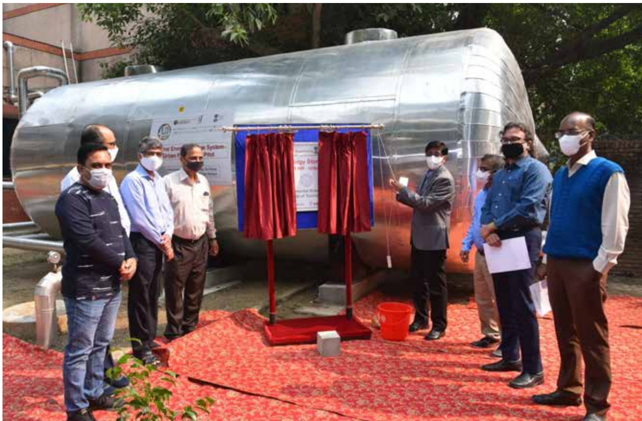
The thermal energy storage system with a 775 tonnes-of-refrigeration heat rate is installed at IIT Kanpur's Centre for Environmental Science and Engineering building as part of the UIASSIST project.
